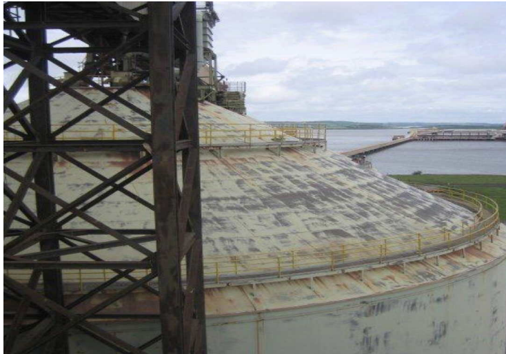
Figure 4: A photograph of the top of one of the Rusal Aughinish silos, with the conveyor belts going to and from ships in the background.
