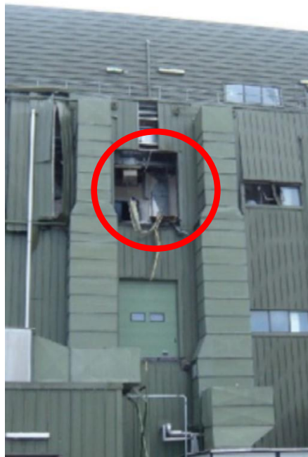
Figure 1: The north side of production Building No. 2 (PB2), post-incident, with the upper roller-shutter door (circled) missing. Image source: Loss Prevention Bulletin
