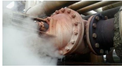
Figure 2: A bonnet / valve body flange with a steam leak. Image not related to this incident. Image source: https://leaksealing.com/
