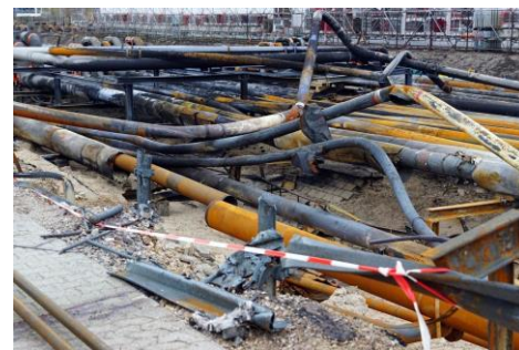
Figure 3: A section of the pipeline trench, post-incident. Image source: Fränkische Nachrichten
