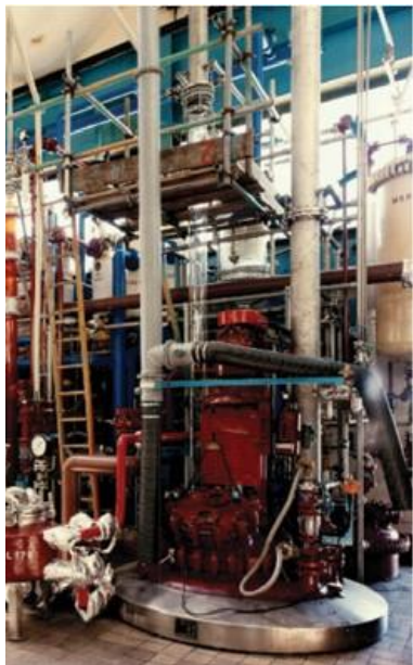
Figure 1: The reactor floor of Building B62, pre-incident. Image source: Loss Prevention Bulletin
