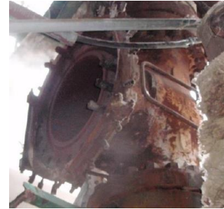
Figure 5: The valve, post-incident, showing the absence of the bonnet. Image source: Team / Total
