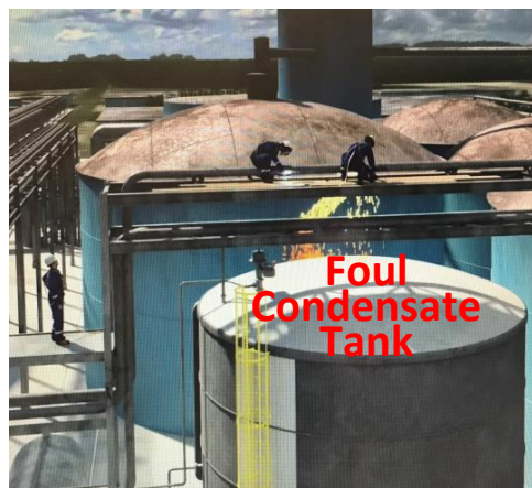
Figure 2: A computer-generated image depicting the hot work being performed on the pipework above the foul condensate tank. Image Source: U.S. CSB (adapted)
