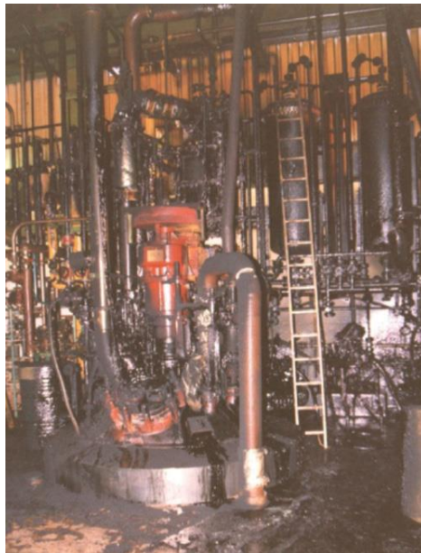
Figure 2: The reactor floor of Building B62, post-incident. Image source: Loss Prevention Bulletin
