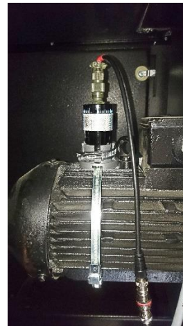
Figure 2. Energy Harvester mounted on an industrial air compressor
